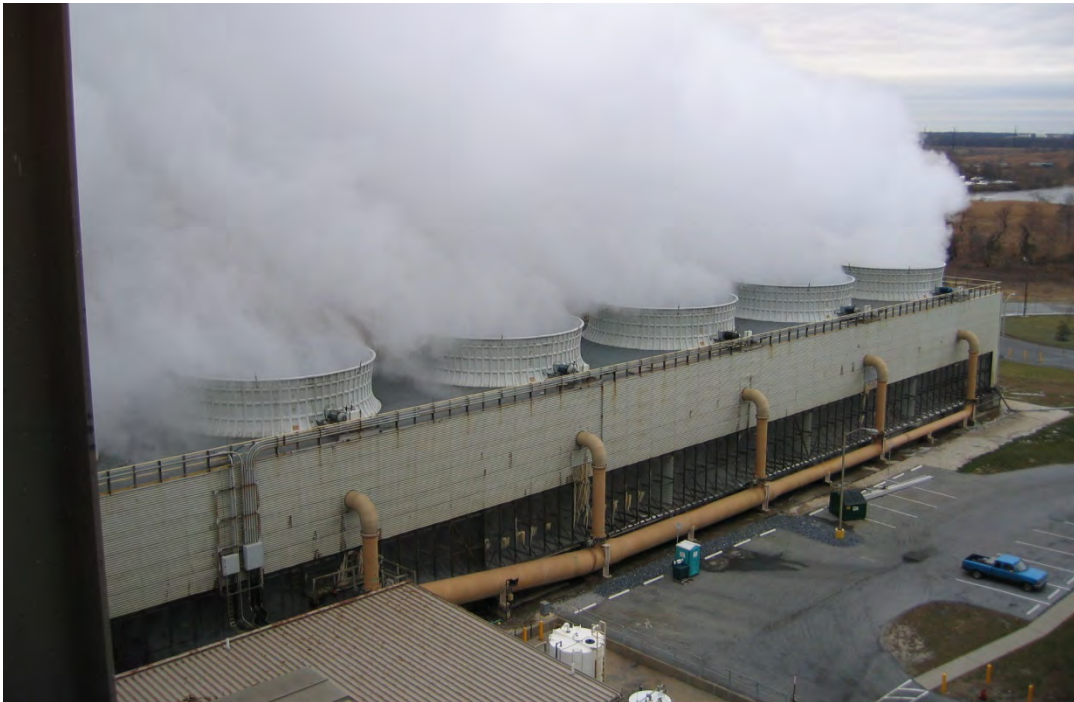
Exhibit 6-3. Mechanical draft cooling towers at Logan Generating Plant, Swedesboro, NJ
